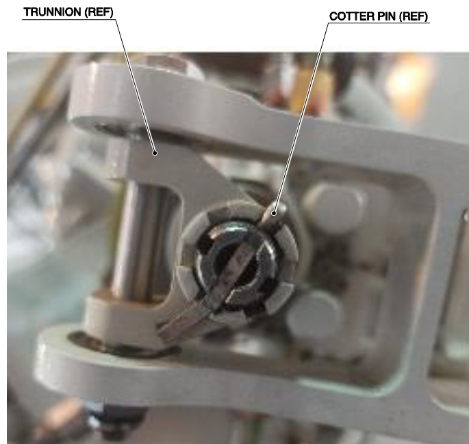
CORRECT COTTER PIN INSTALLATION WITH NO SIGN OF ROTATION VIEW B1
