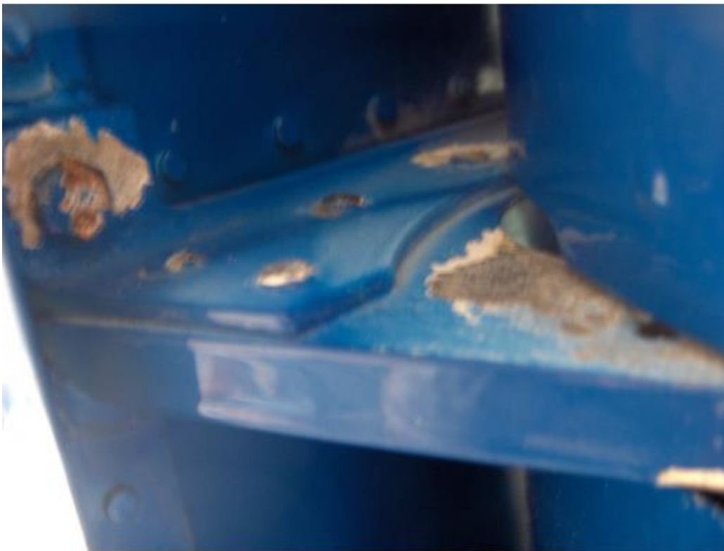
Hinge Corrosion Example
