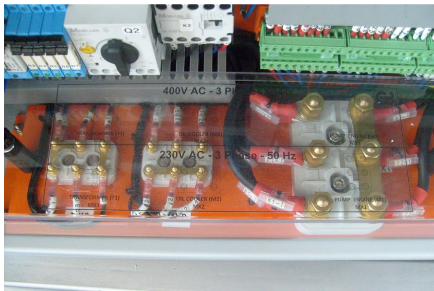
Terminal block for voltage change
