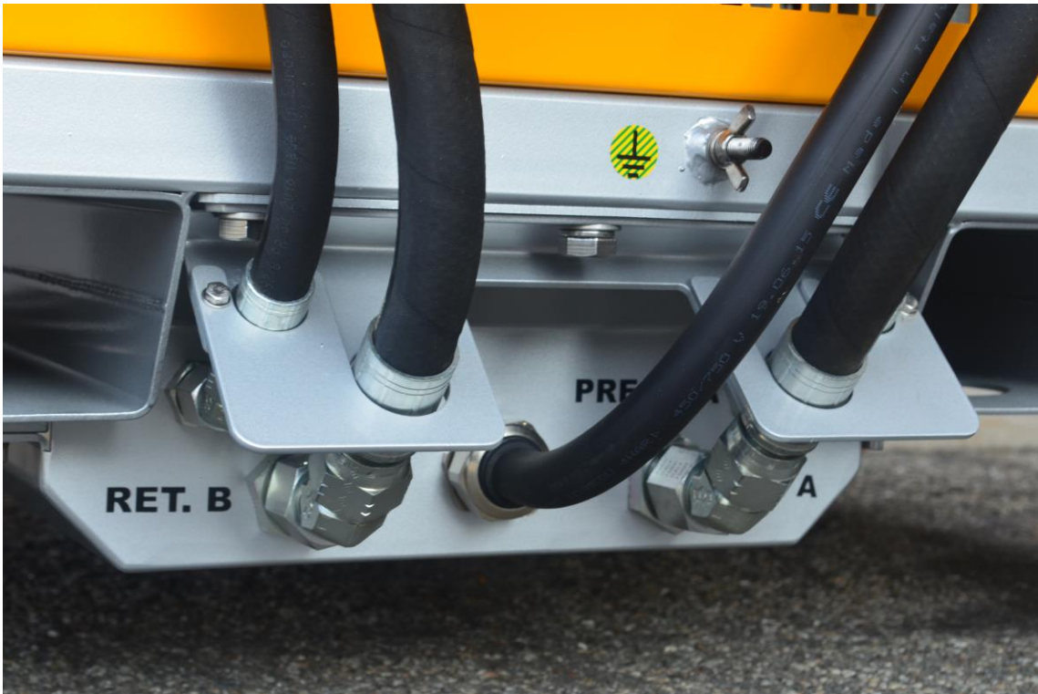
Delivery and return flexible hoses, test bench side
