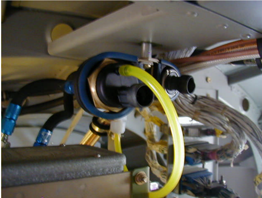
Figure C- 12: Pitot/Static Installation on 1900D
