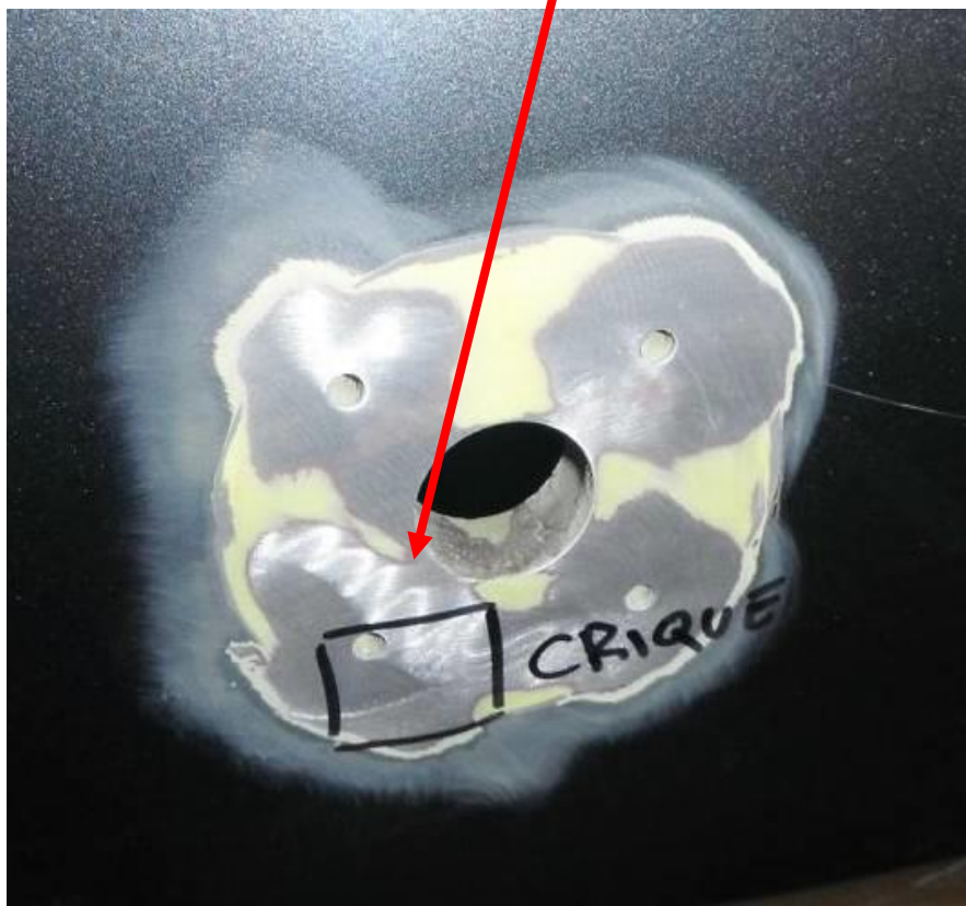
Figure 4 (Examples of cracks)
