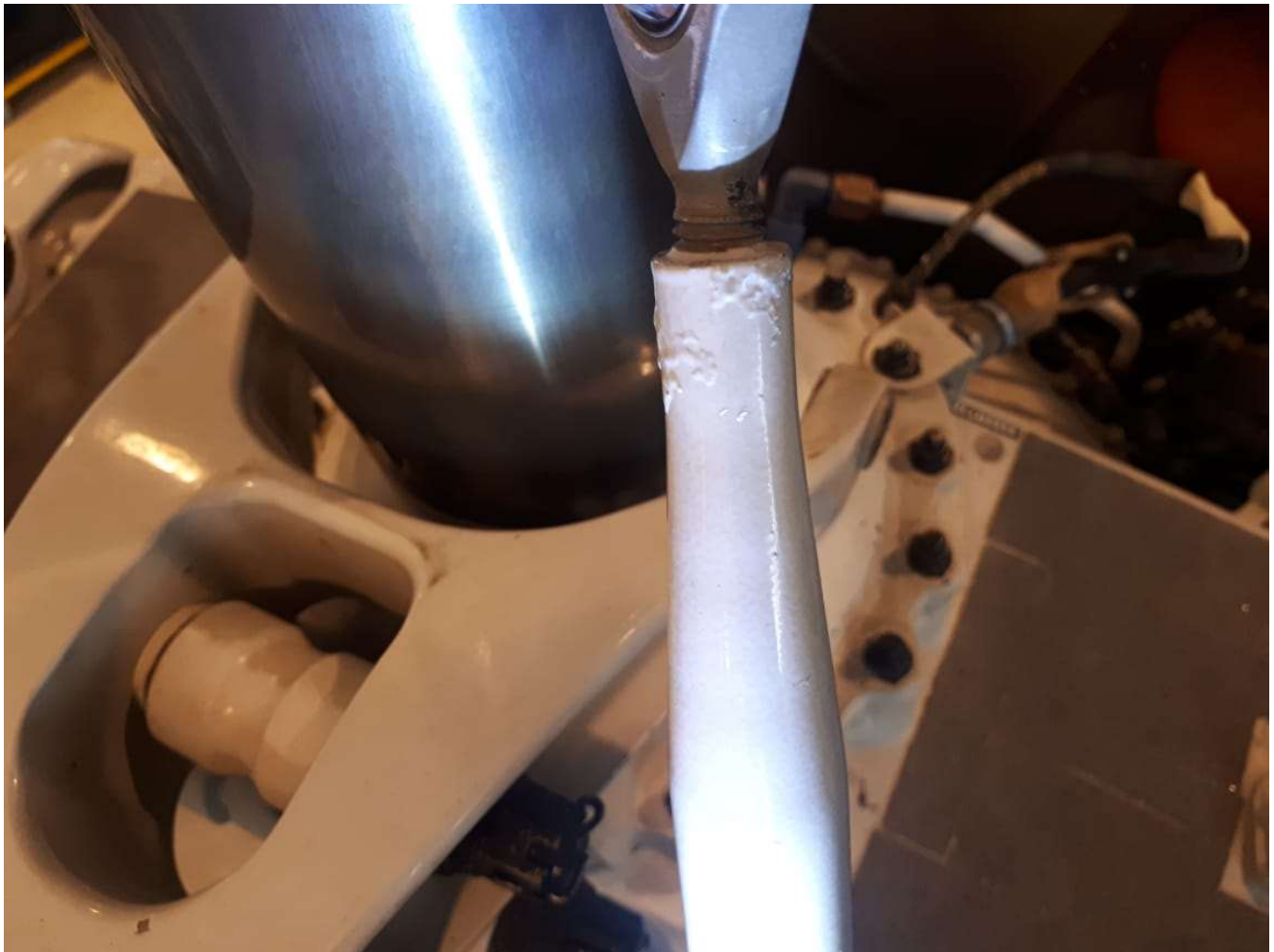
Figure 2 – Corrosion on Swashplate Cyclic Input Tube
