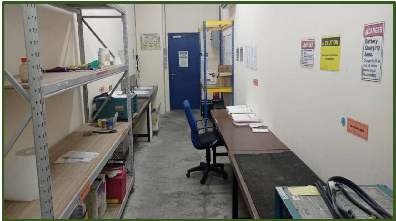
A1: FROM INSIDE VIEW LEAD ACID BATTERY WORKSHOP ROOM (FROM THE BACK WALL)
