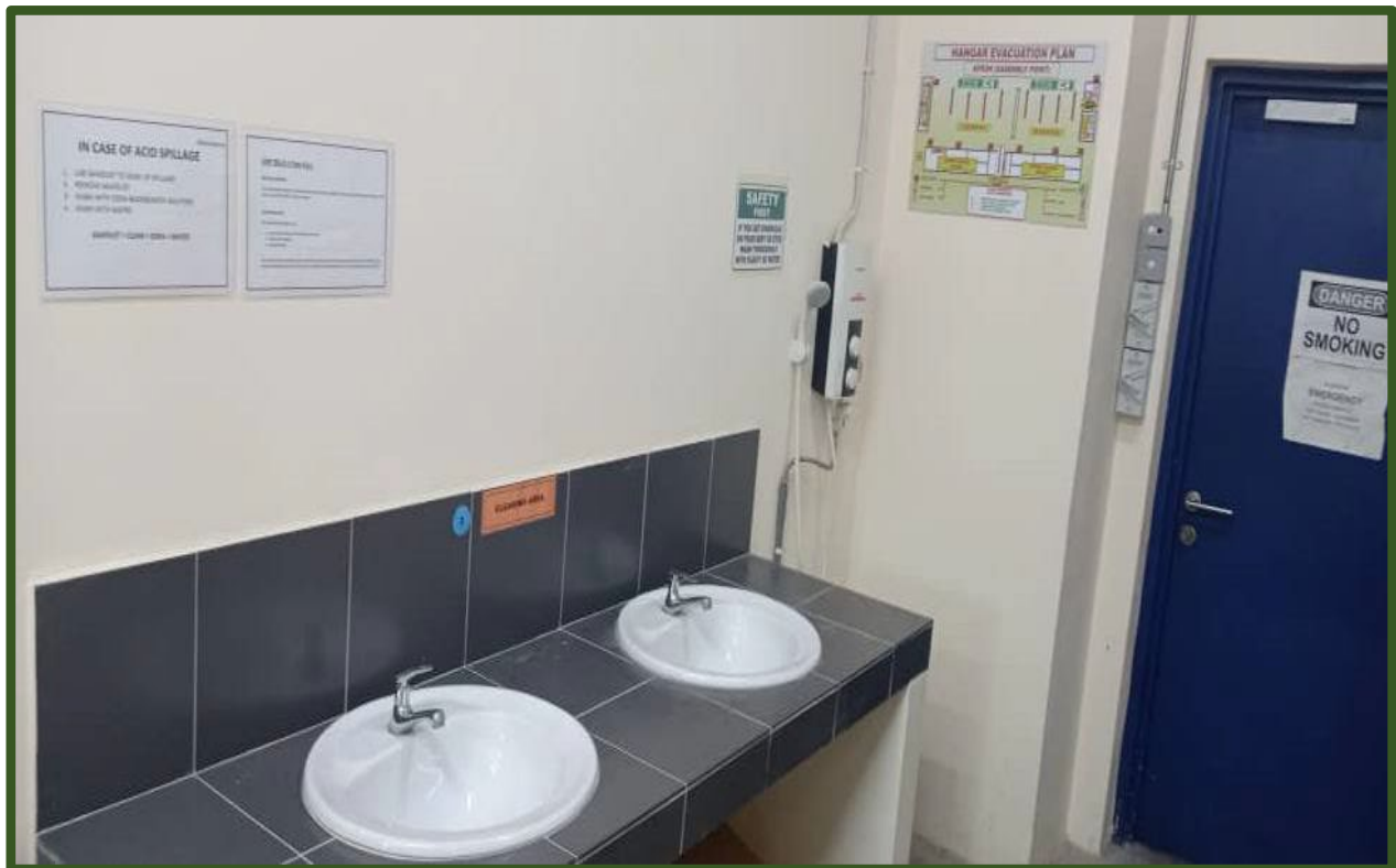
A2: INSIDE VIEW LEAD ACID BATTERY WORKSHOP ROOM (POSITION OF THE SINK AND SAFETY PLACARD)
