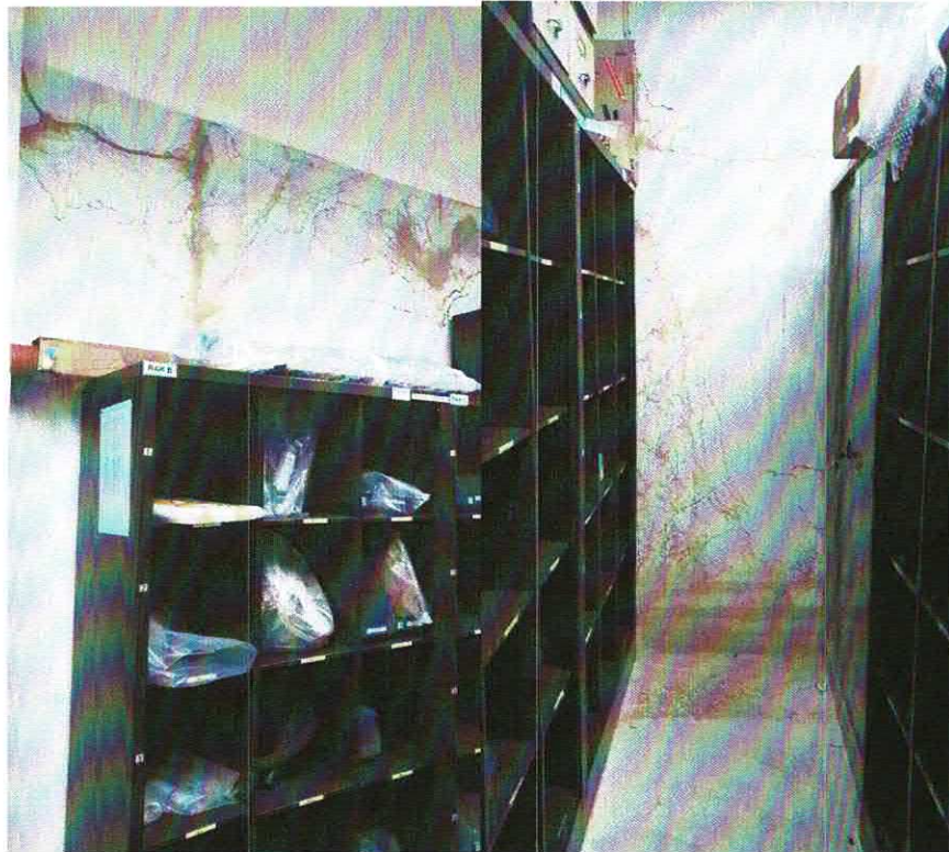
Figure 5: Holding Room Condition
