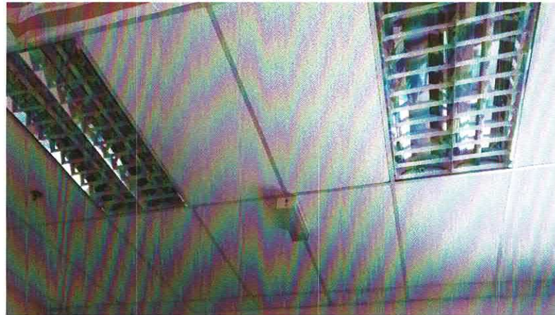
Figure 3: Lighting are broken.
