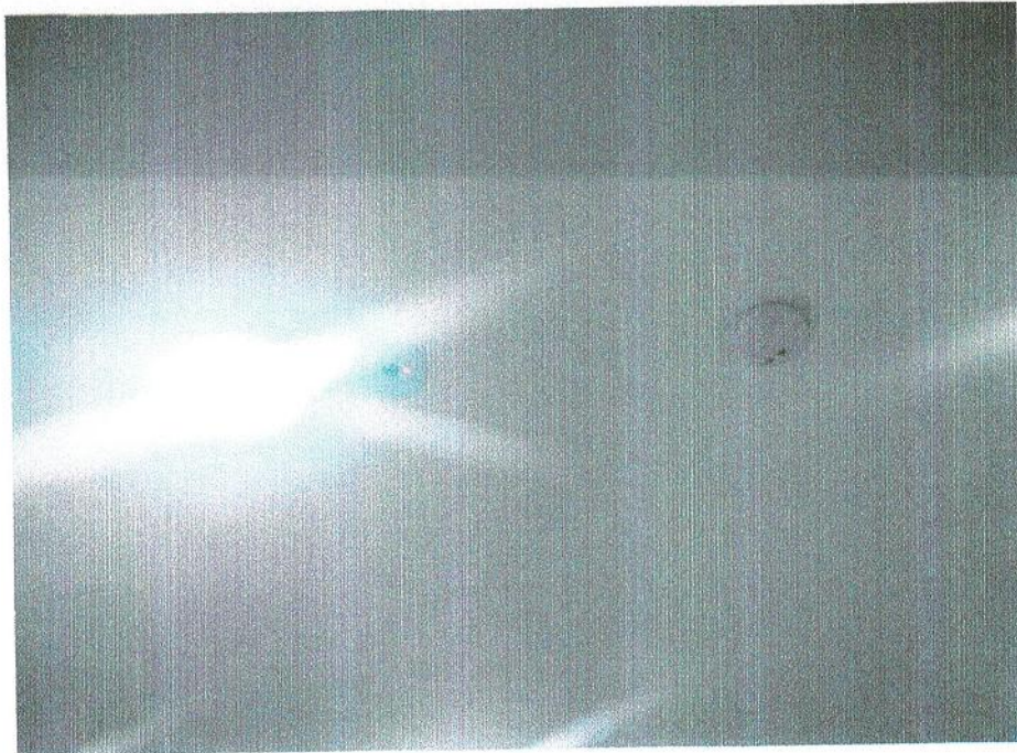
Image 1 : Emergency light and smoke detector
