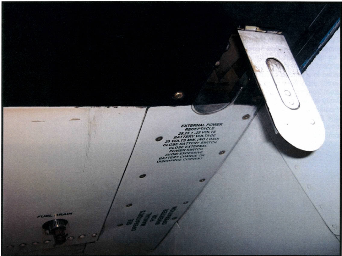
External Power Connection
