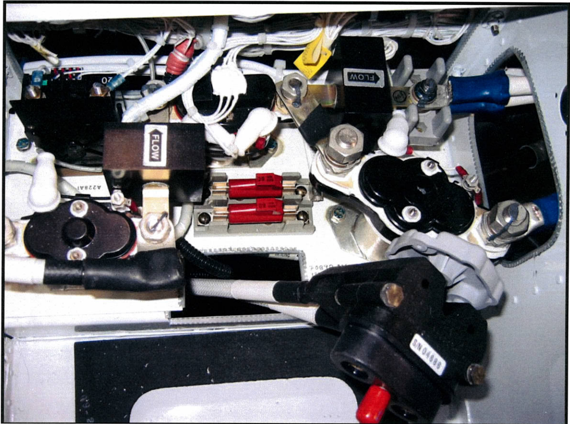
RCCB- Battery Contactor- Battery Bus Tie- Right Bus Tie- Hall Effect Sensors- Ground Power Contactor
